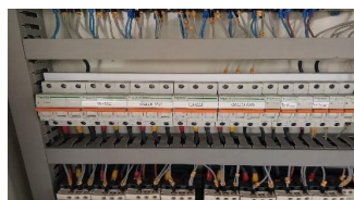
Gambar 2.21 MCCB instalasi panel
