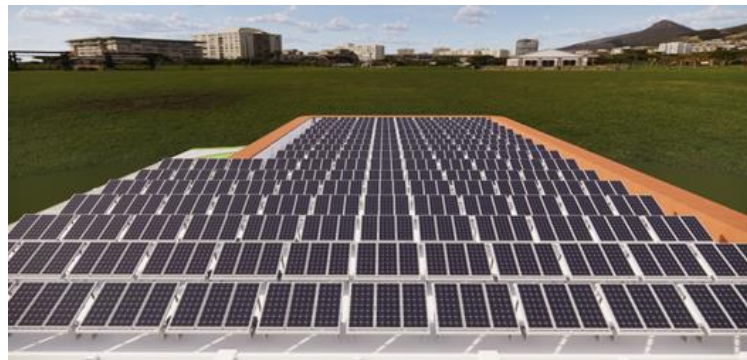
Gambar 5. 10 The Grove solar system
