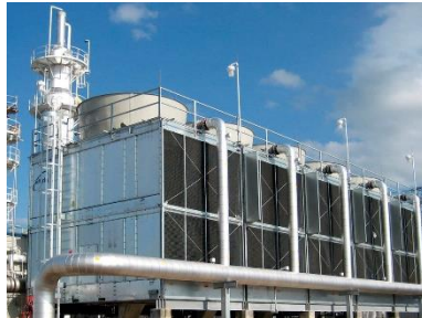
Gambar 4. 34 Cooling Tower (CT-01)
